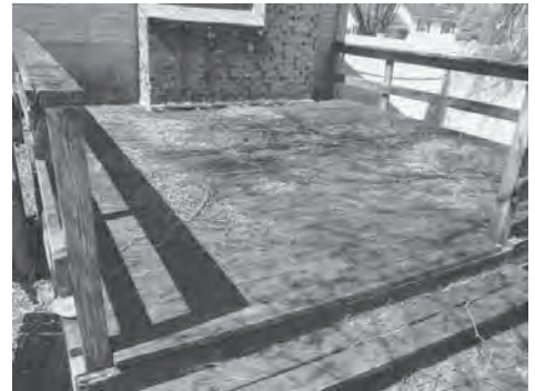
deck, poor condition
